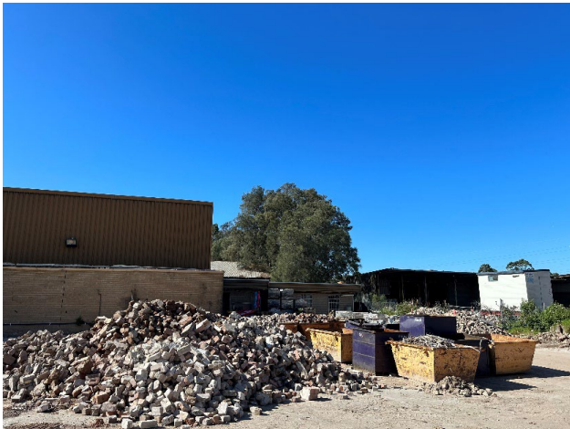
Figure 28 – Existing structures at the site – taken from the rear of the site looking east
