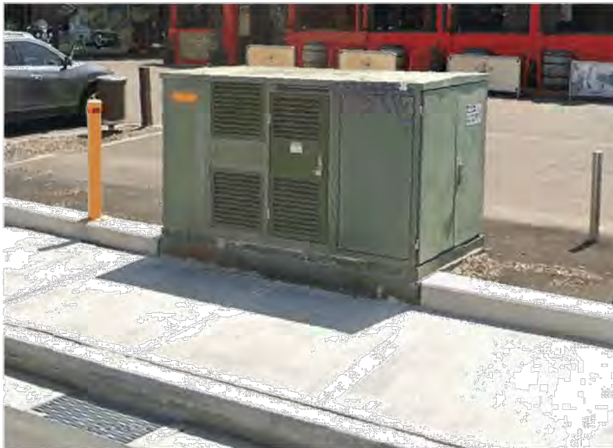
Figure 1 Typical existing Ausgrid transformer kiosk, as the basis for the JUMP charging stations
