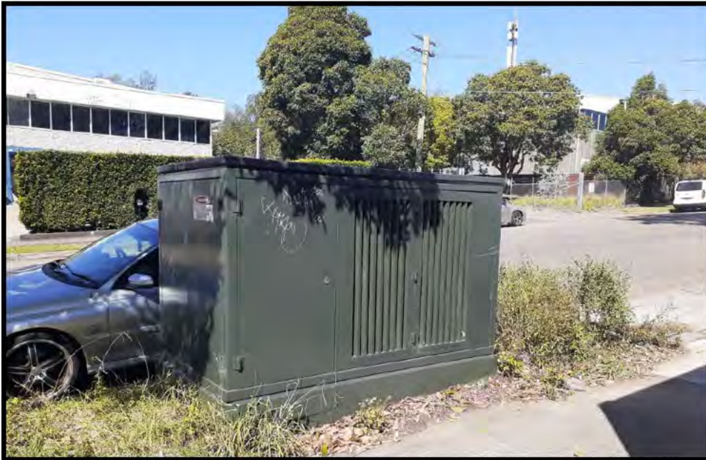
Figure 3: Existing substation kiosk
