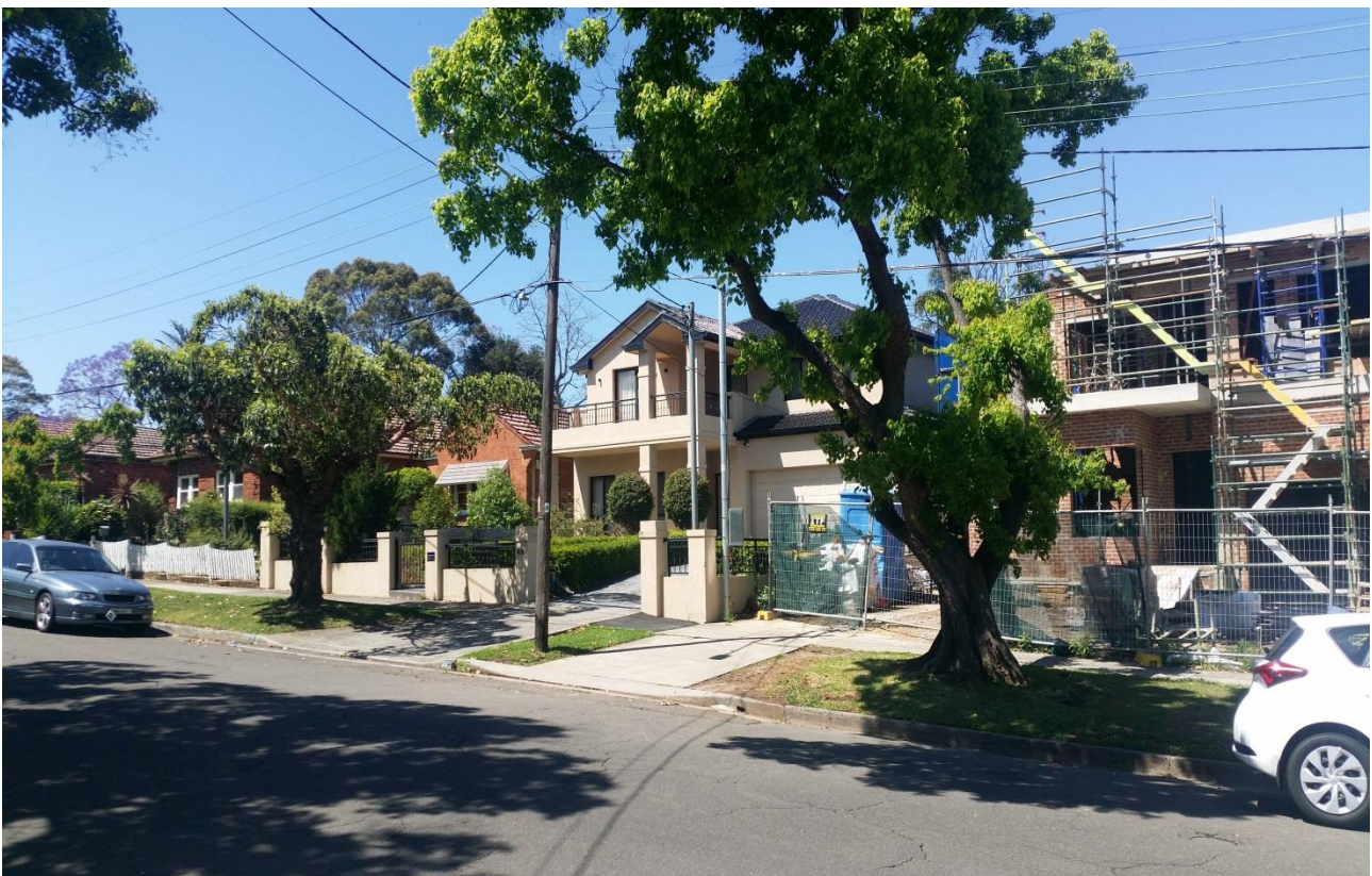
Figure 3: View from subject site looking east showing flat roof two (2) storey dwelling under construction at No.50 Myrna Road
