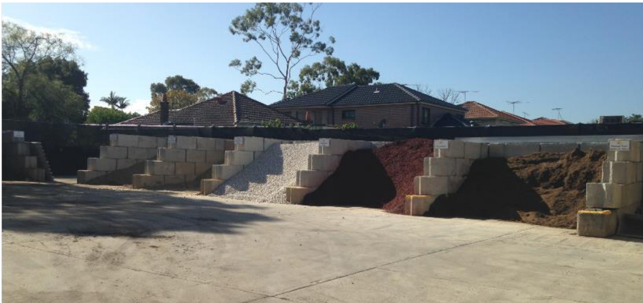
Figure 4: View of unauthorised works within the subject premises with no acoustic barrier.
