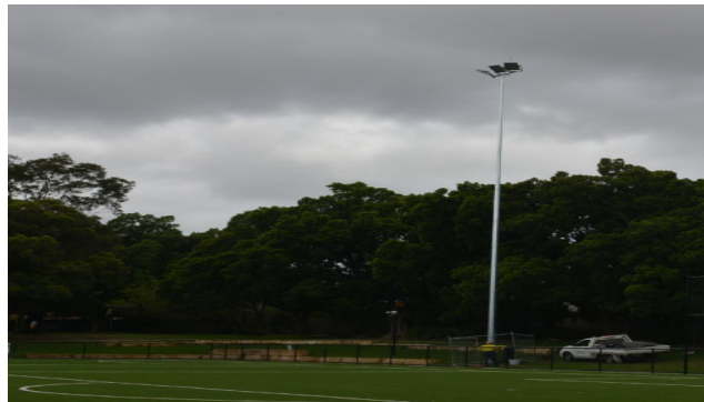
Sports floodlighting (synthetic fields) condition is rated as Excellent.
