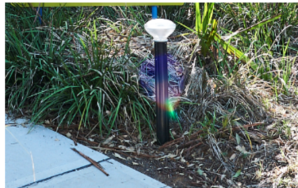
Bollard Solar LED lights are rated as Good
