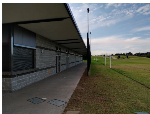
Amenities building and sports lighting were built in 2018. The condition is assessed as excellent
