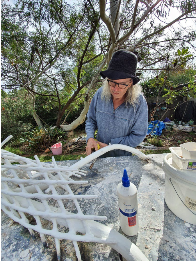
Construction of "The Fallen Angel" during the first covid lockdown in Sydney, 2020
