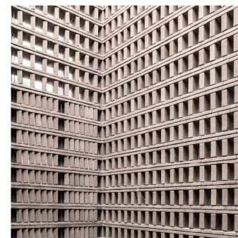
BL2 - NATURAL LIGHT COLOURED FACE BRICK OR EQUIVALENT SIMILAR PERFORATED WALL LOCATION: SCREENING & WINDOW SHADING AT NORTH & WEST ELEVATION
