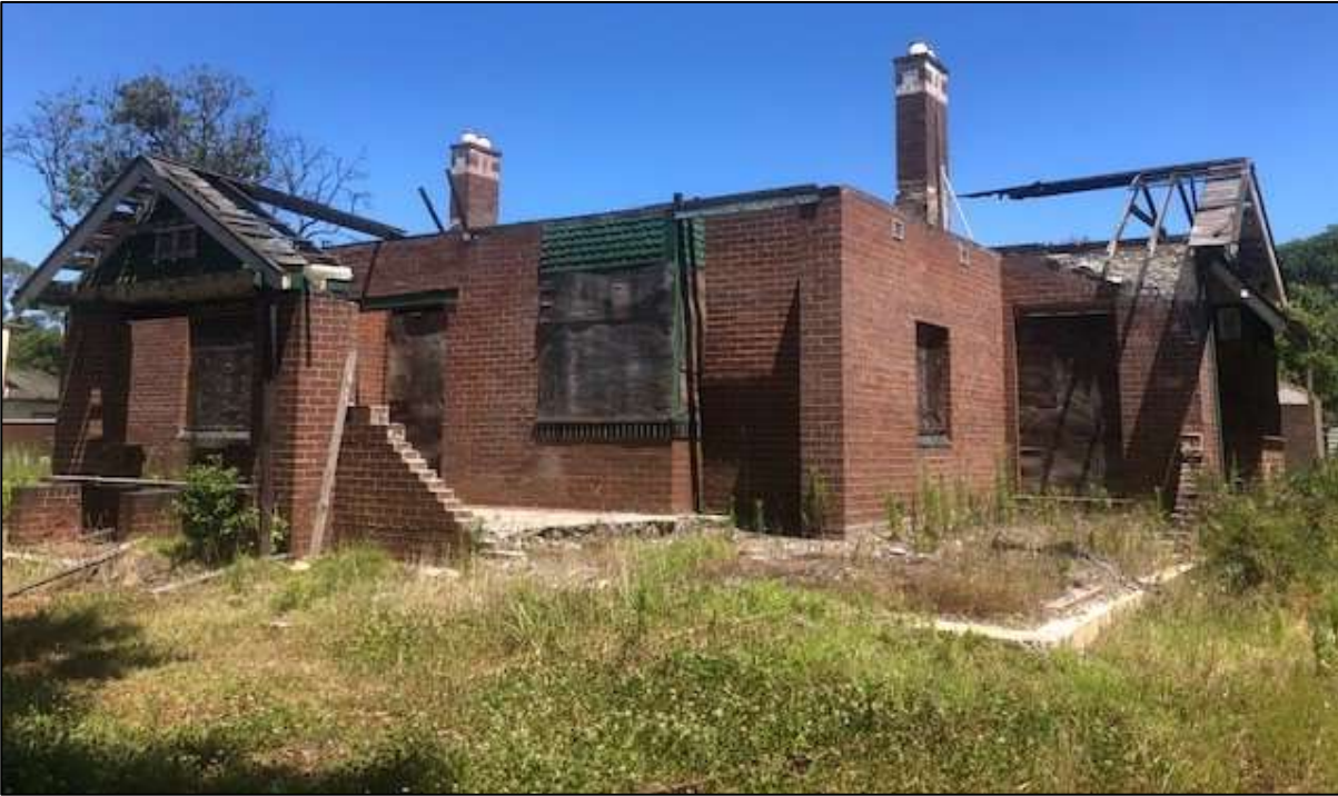
Figure 10: Heritage dwelling in its current dilapidated state from Burlington Road.
