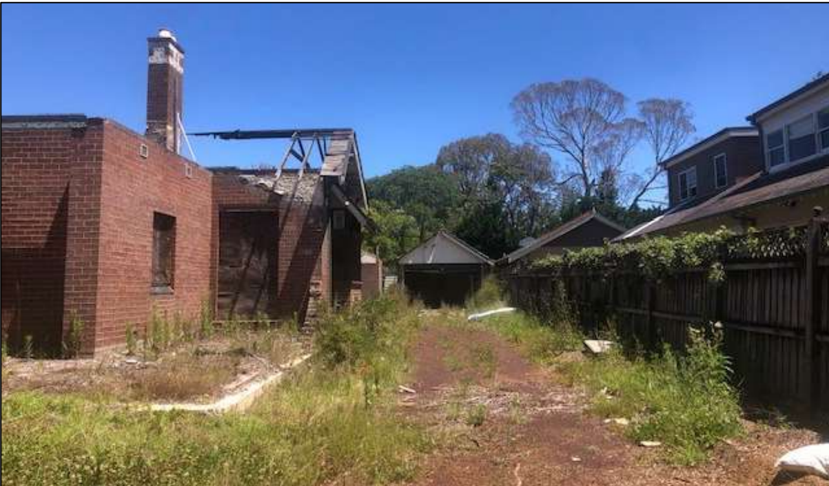
Figure 11: Remaining western wing and western driveway leading to detached garage. The garage is a later 1940s-1960s addition and is not included as part of the heritage listing of the site.
