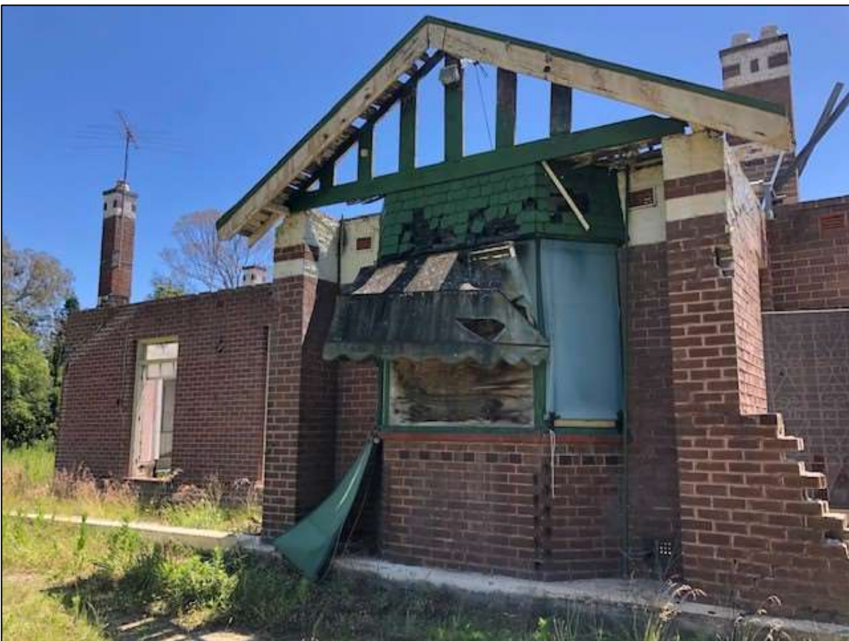
Figure 15: Dilapidated eastern wing with bay window proposed to be restored.
